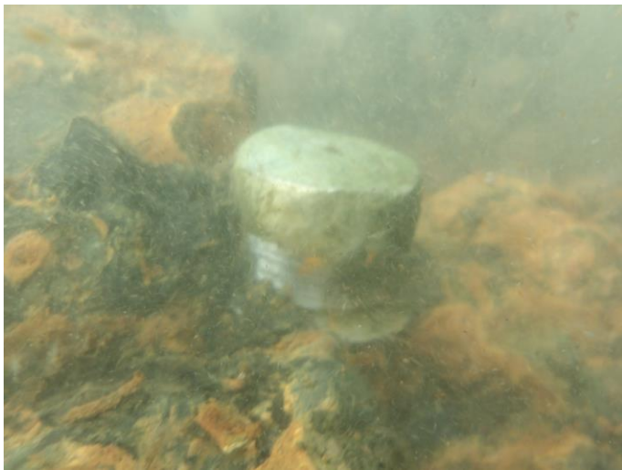
Underwater photo we believe of the valve stem top protruding through the operating wheel.
