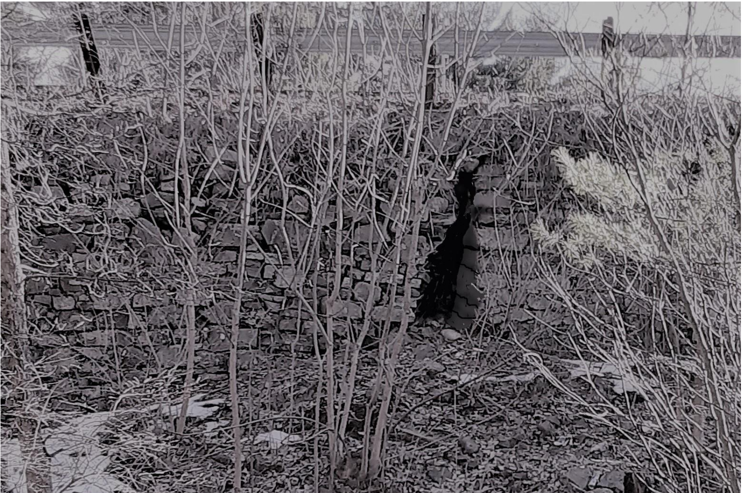
Six-foot hole in west face of dam wall. Stones to the left of the hole appear to be collapsing.
