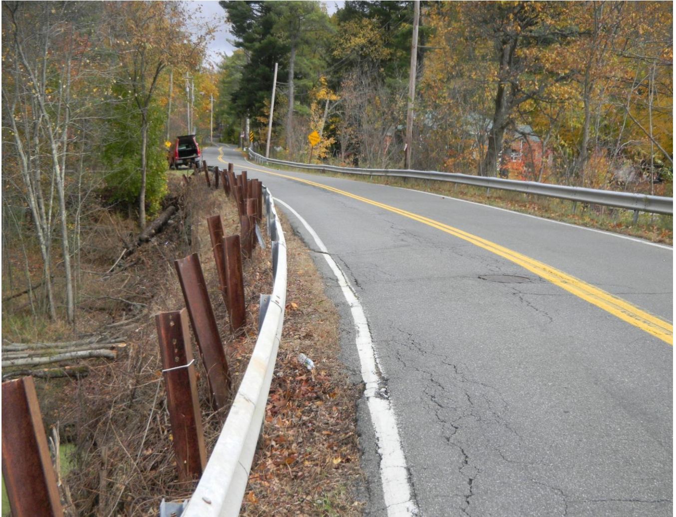
Stress cracks in road atop dam
