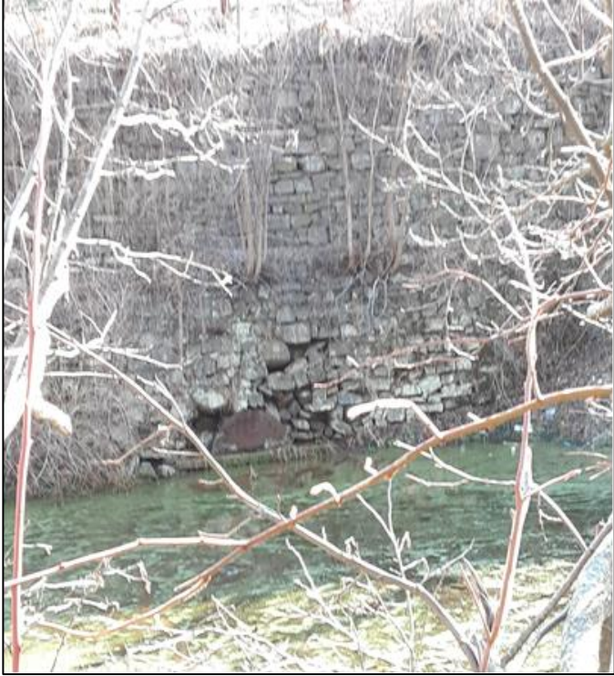
Loose rocks around outlet pipe
