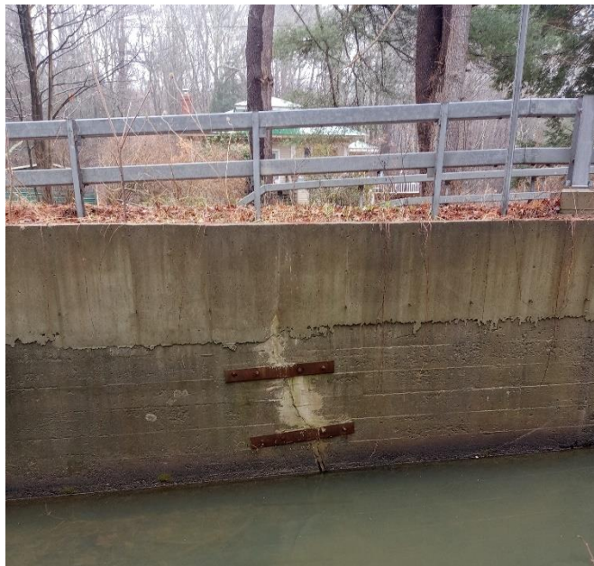
Old repair of Spillway wall may need attention.
