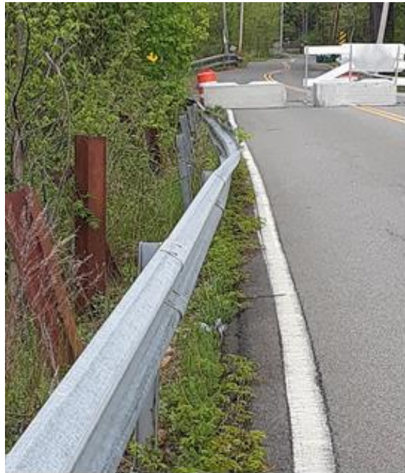
On closed portion of road, guard rails and supports are separated and unstable.
